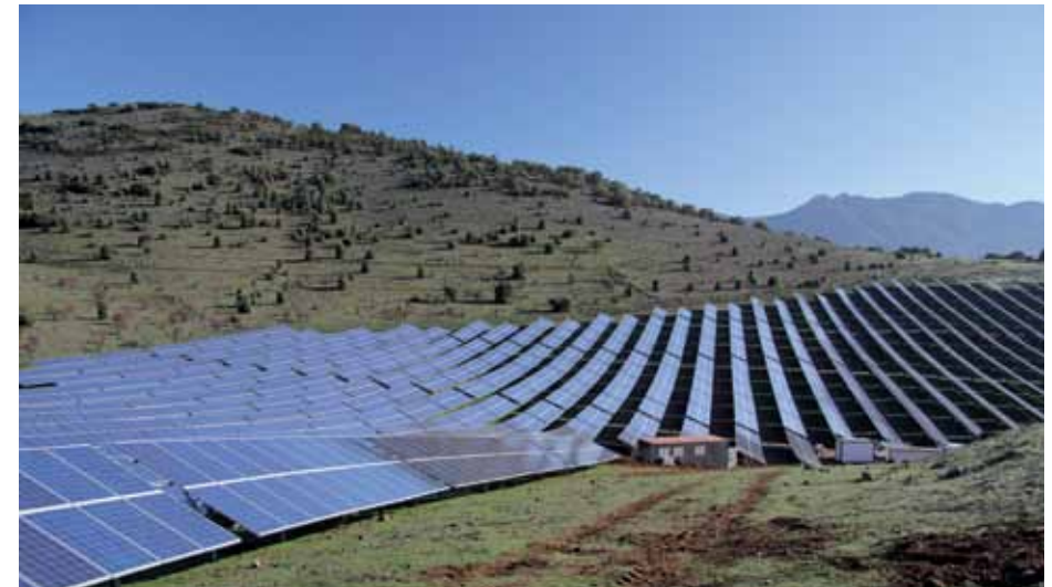
Korsika Verde | Korsika - France System: 2,6 MW | T-Rack System
