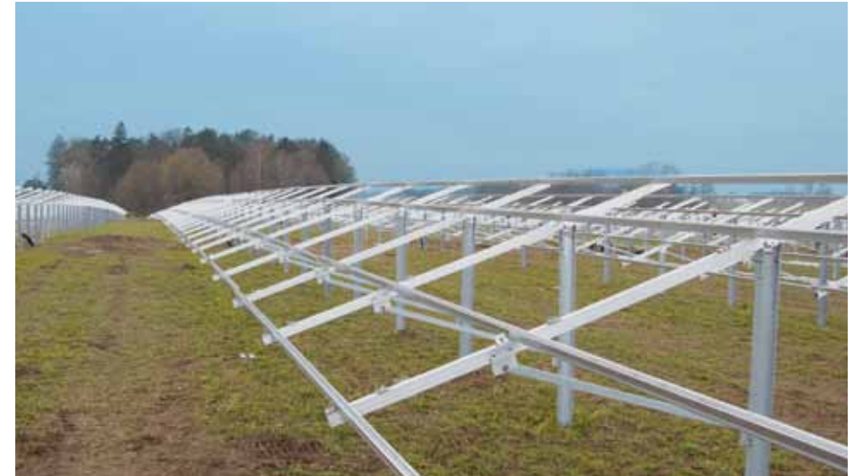
Krannich | Nierpars - Germany System: 3,942 MW | T-Rack System
